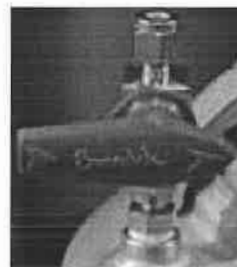
Figure 4.6 – Example of a Closed Valve
